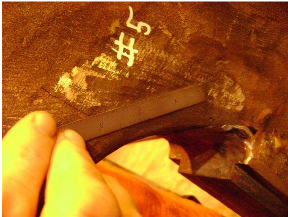
Figure D.41. Indication 5 (after 6 million cycles and grinding)
