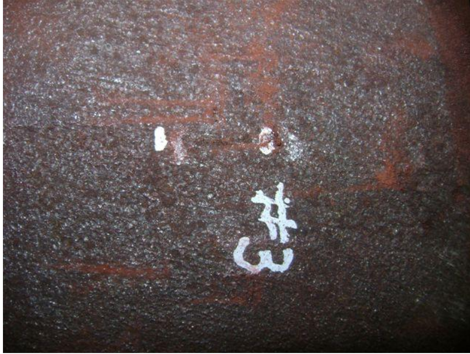
Figure D.28. Indication 3 (top of pedestal after 2 million cycles)
