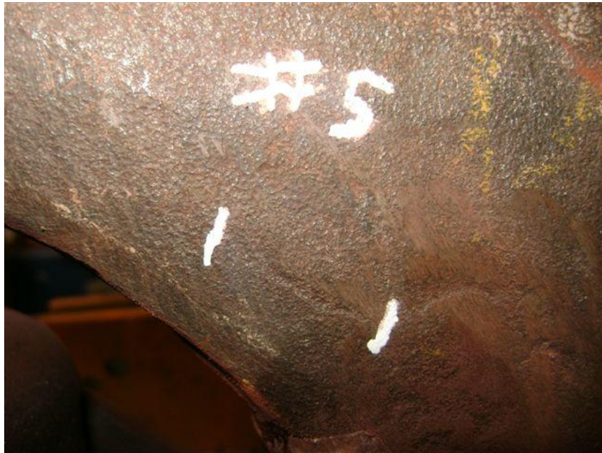
Figure D.35 Indication 5 (after 4 million cycles)
