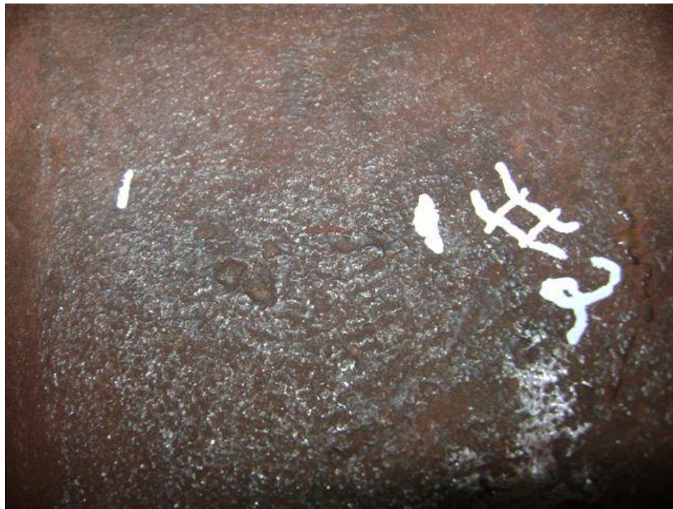
Figure D.27. Indication 2 (top of pedestal after 2 million cycles)
