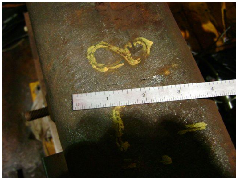
Figure D.25. Indication 1 at gage 8 (top of pedestal after 2 million cycles)
