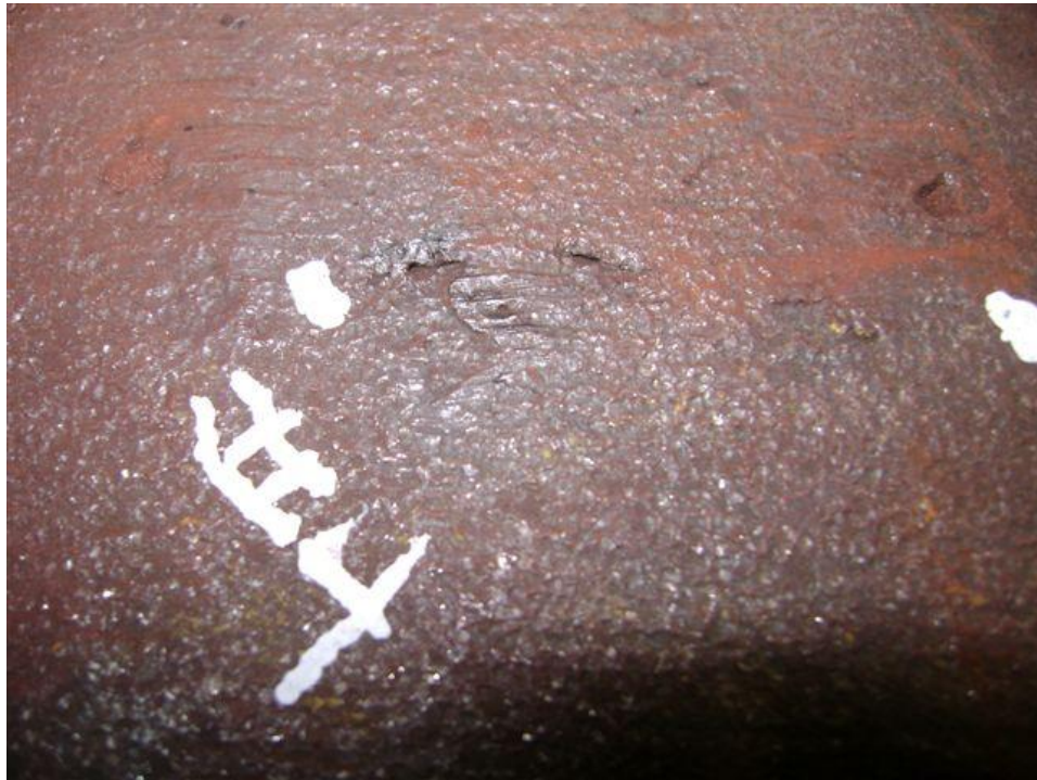
Figure D.29. Indication 4 (top of pedestal after 2 million cycles)
